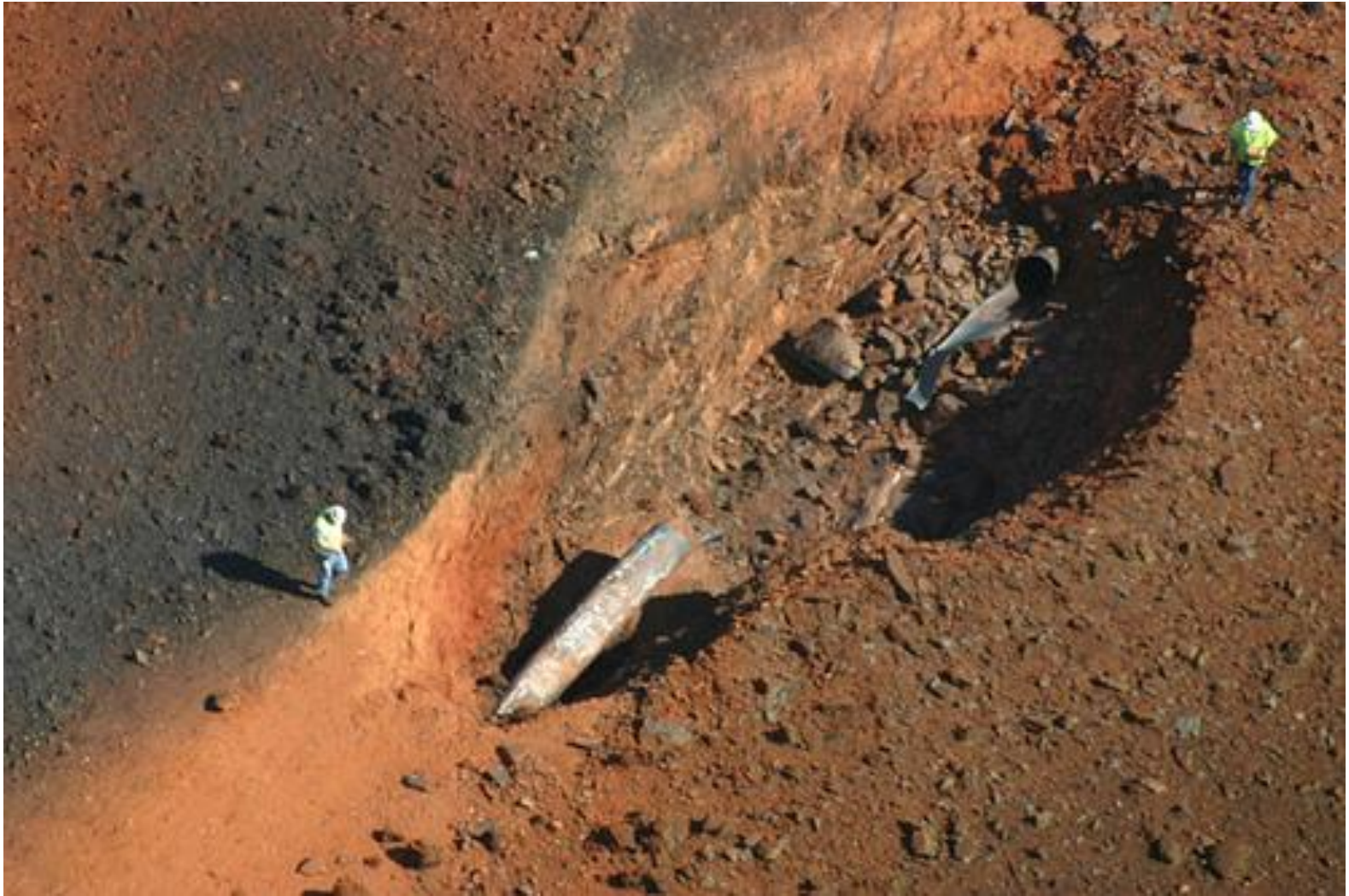
Crater from Appomattox pipeline failure
